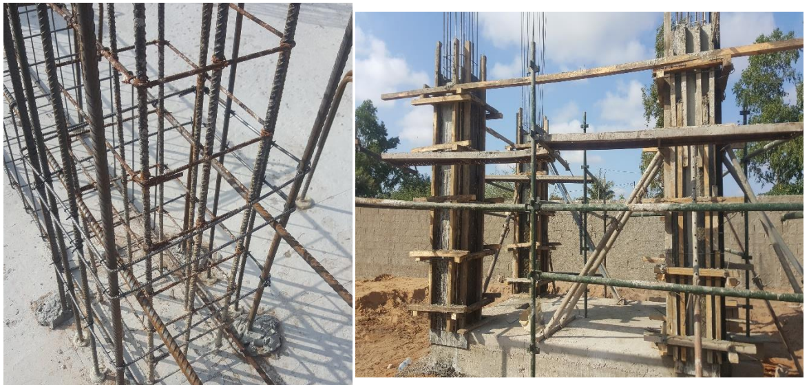
Figure 13. Junction between frame and iron wire, and formwork of water tower pillars
