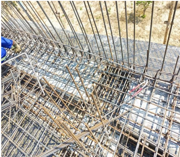
Figure 7. Elevated deposit box slab frame
