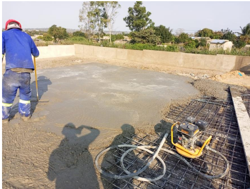
Figure 9. Top view of partial concreting of the slab of the manager's house
