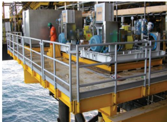
Figure 13. Offshore Environment of Methanol Injection Pump Packages -7033 in full operation.
